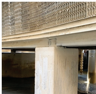
Image 2. Due to operational issues, the plant was unable to respond to the early deposit stress warnings. As a result, an iron-silica deposition event occurred which fouled the cooling tower and condenser and forced shutdown for remediation.
